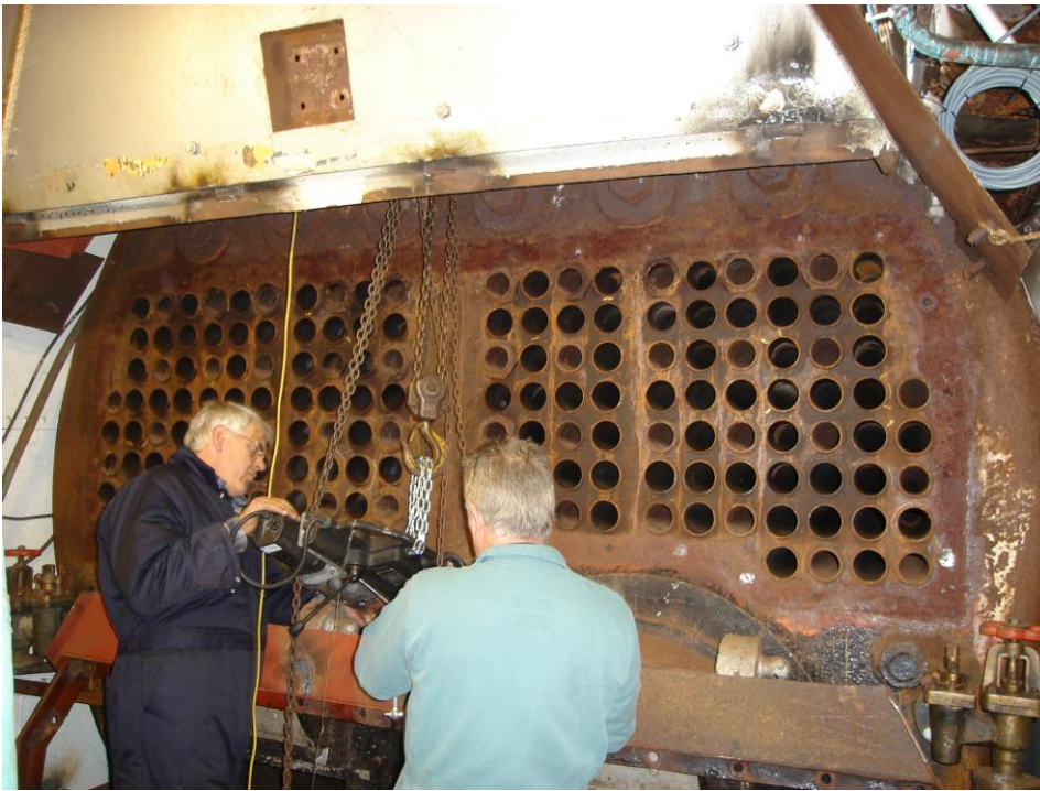
The exposed fire/smoke tube ends in Lydia Eva's Scotch Return Tube boiler built in 1961. Lydia Eva is a preserved steam drifter, launched in 1930 and now based in East Anglia in the ownership of the Lydia Eva and Mincarolo Trust.
